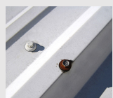
Fasteners & washers showing signs of corrosion
