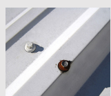
Fasteners & washers showing signs of corrosion
