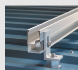
Corrosion around fixtures and fittings*
